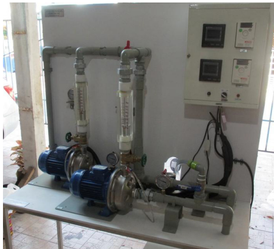
Fig. 1: The experimental setup: pumps and connections.
